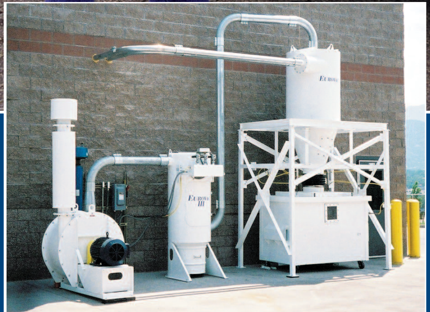
Centrifugal Eurovac multi-stage pump with multiple cartridge filters and automatic compressed air "PulseJet" cleaning (with pre-separator depositing debris directly into dumpster).
