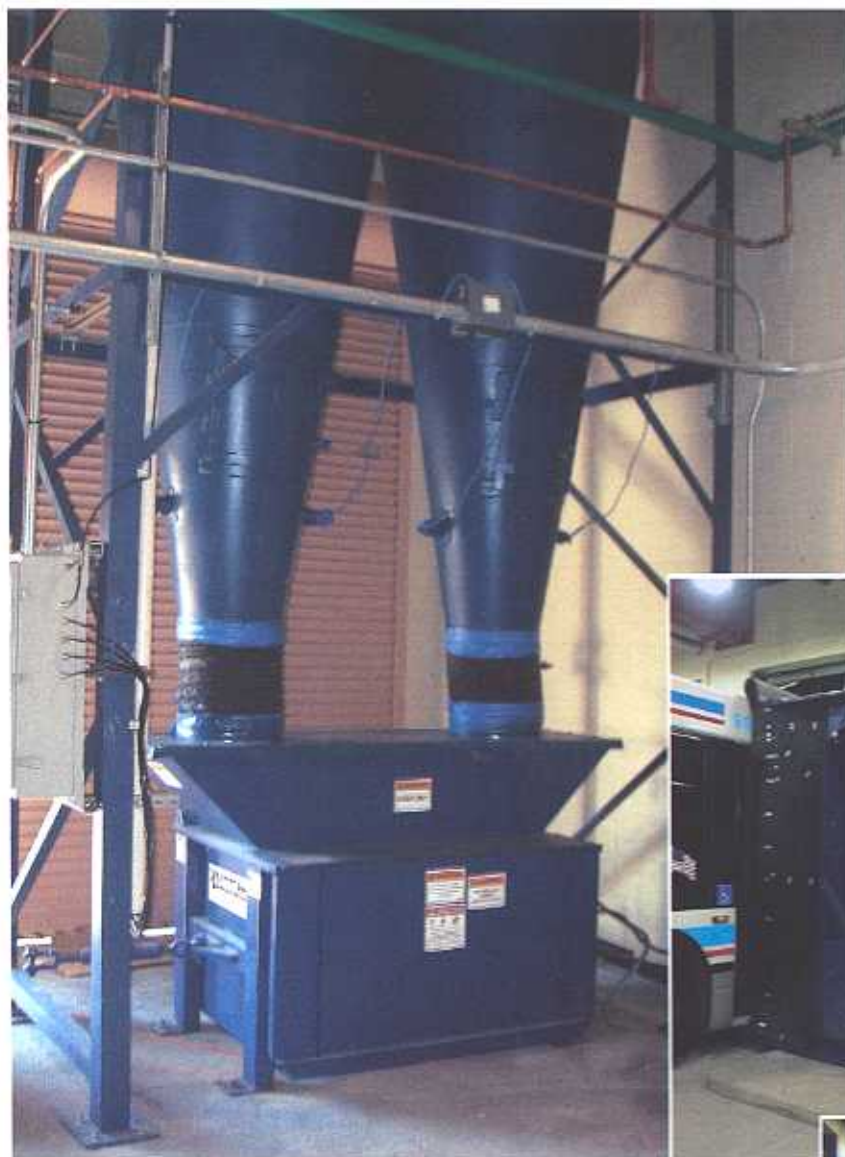
Single-lane cyclone separator with compactor/dumpster
